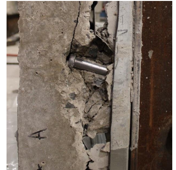
Localized damage around the stud
